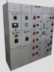
AMF WITH MCC PANEL
