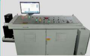
BLOCK MAKING MACHINE PANEL
