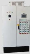
CURING CHAMBER PANEL
